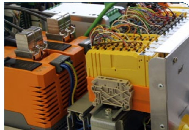
Advanced controller inside
