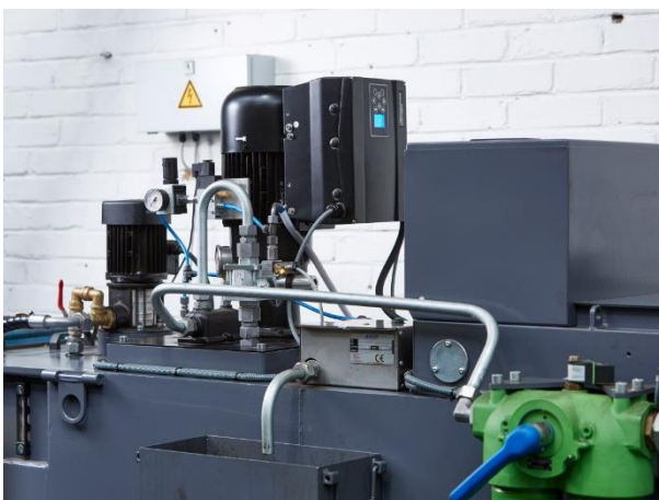
Integration neue KSS-Anlage
